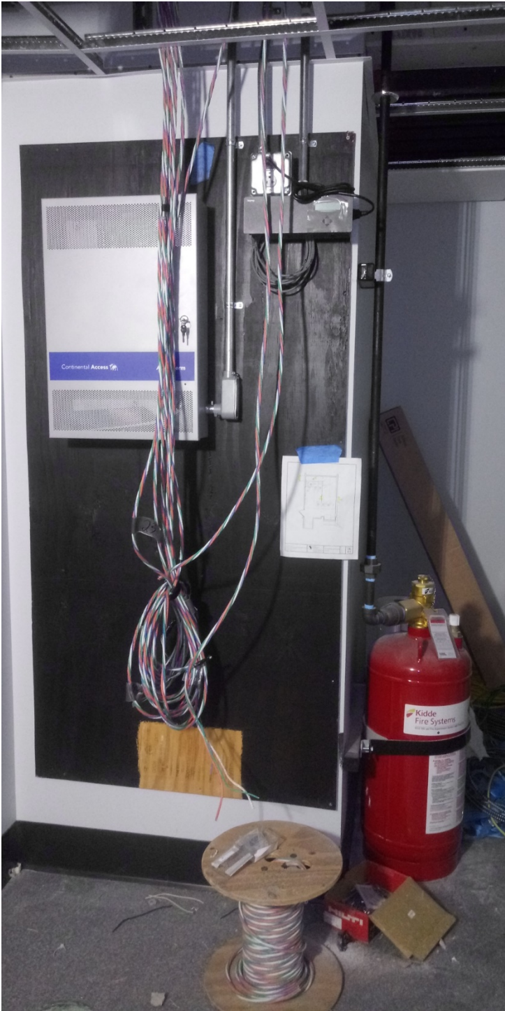
Server Room 122 – Clean Agent Control Panel & Sound Masking System installation continues.
